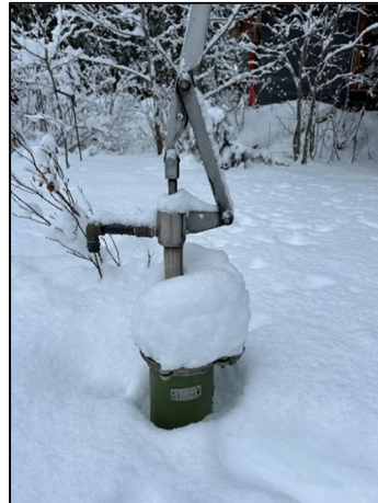
Photo 18. View of water pump at well location.
